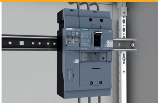
3VA1 molded case circuit breaker, 160 A, with TMTU and side mounted RCD – installed in a distribution board.
